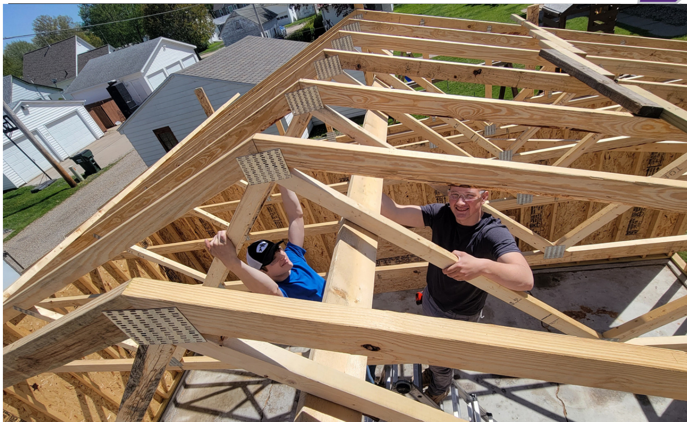
Students in Kyle Krieger’s Construction Trades class work on a three-car garage for an area resident. They started the project this past spring and completed it Nov. 1.
